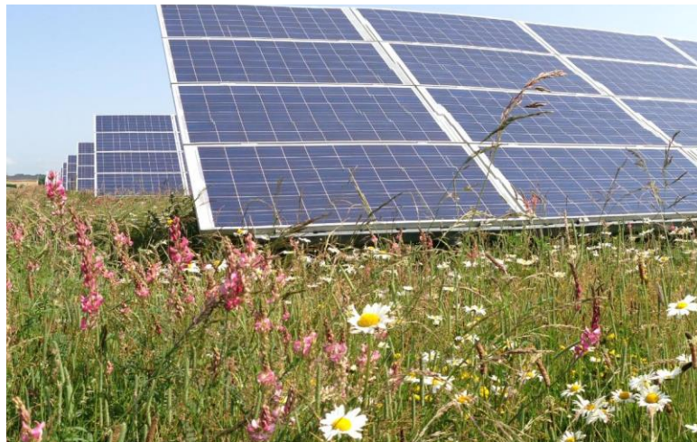
Connexus and Fresh Energy pollinator friendly PV project, Minnesota
